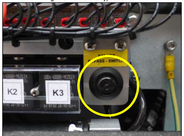
Fig. 4.3.4-6: Failure bypass switch
