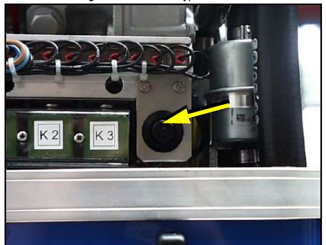
Fig. 8.9.2-1: Failure Bypass Switch
