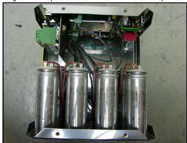
Fig. 6.11.3-2: Opened AC Control Box from Panda 30 upwards
